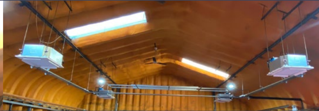
Quadruple Installation configuration
