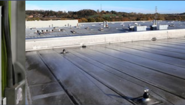
Roof view of some A/C assets
