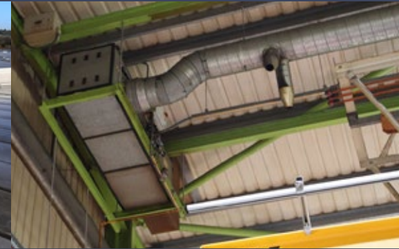
Air Handling Unit
